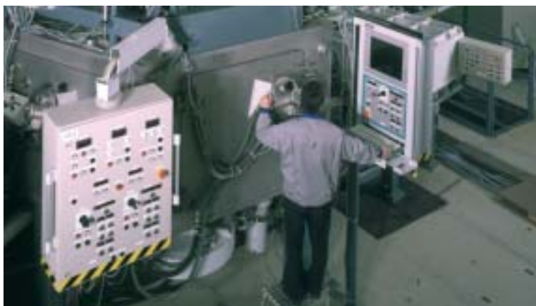
Local operation panels.
