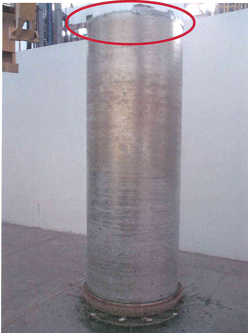
Figure 2 - unacceptable: top with crown (acceptable surface)
