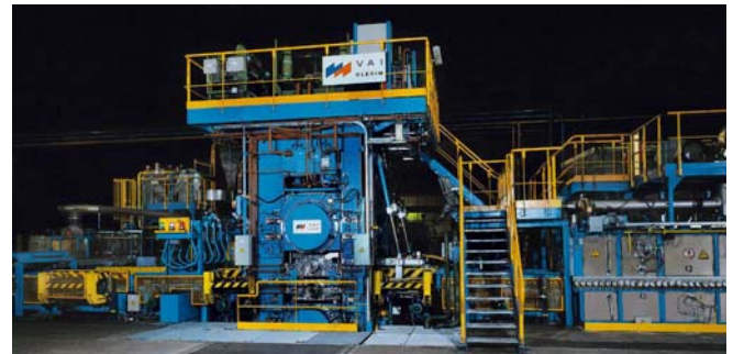
Hot rolling mill
